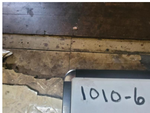
1010-6 12"x12" Floor Tile/Tan (2% Chrysotile) Mastic/Black (3% Chrysotile) Interior Kitchen/Bottom Layer (Appx 190 sq ft)
