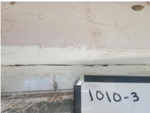
1010-3 Caulk/Tan (4% Chrysotile) Typical Exterior Windows
